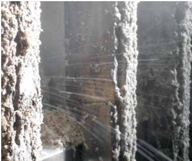
Fig. 5: Spurts in the enbloc perforated plates (type A) following the opening of the holes clogged by fine pulp
