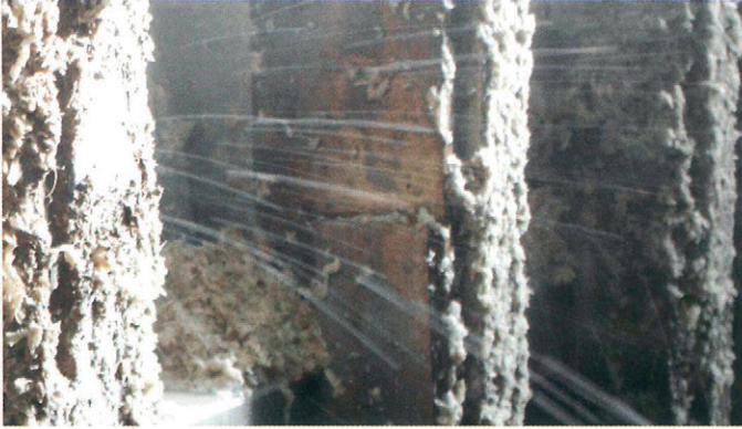
Figure 5: Spurts of water from the enbloc perforated plates (type A) following the opening of the holes clogged by fine pulp
