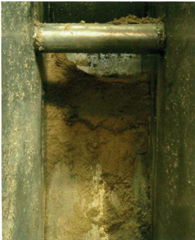
Fig. 9: Deposit of sand on the filtering cage
